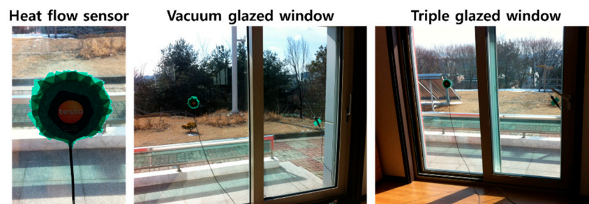
Figure 9. Installed heat flow sensors for each window.
