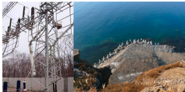
Figure 9. On-site testing of a 220 kV 13.3 km long XLPE cable circuit: The damped AC system HV300 is connected to one of the cable section phases (left) and the transition point between land and submarine cable (right).
