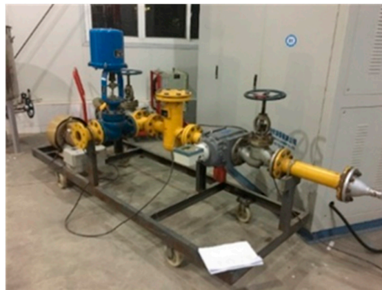
Figure 5. Air supply unit.
