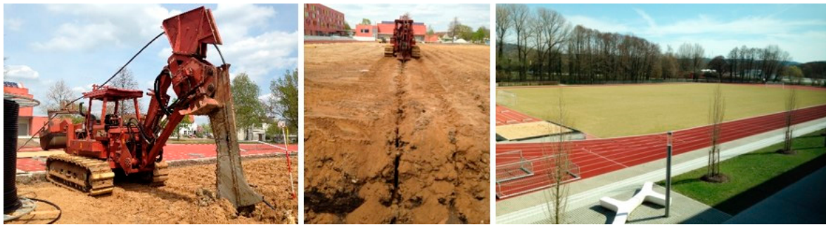
Figure 2. Installation ( left and middle ) and finished Agrothermiefield under the sports field ( right ) (Pictures: EGS-plan).
