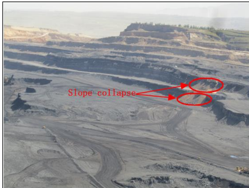
Figure 8. Two collapses occurred on the north slope in the Anjialing open-pit mine.
