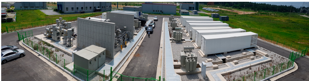
Figure 11. KEPCO Gochang BESS demonstration system.
