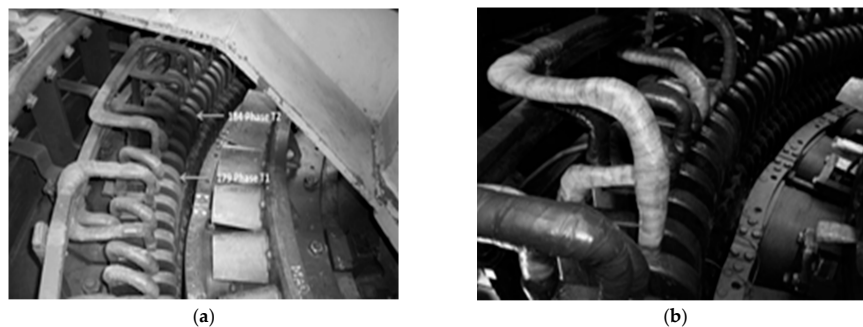
Figure 4. Fault indication and mitigation in the stator winding of generating unit (GU) #1: (a) fault indication; (b) fault mitigation.
