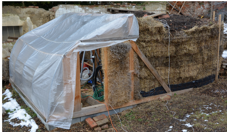
Figure 13. Composting bioreactor before final connection of heat recovery and temperature measurement circuits.
