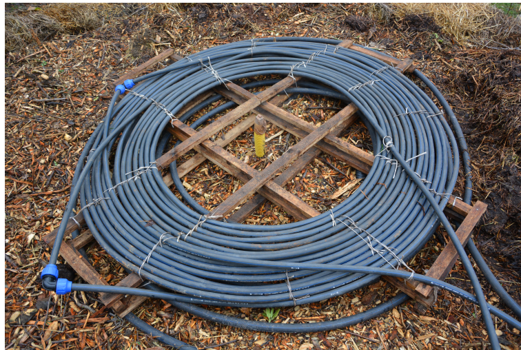
Figure 4. Prototype of the heat exchanger: L-shaped fittings connect three shorter sections of the pipe forming a total length of 61.2 m. Wider LDPE pipe visible underneath the exchanger is a potential second heat exchange loop—it had not been used in this experiment.
