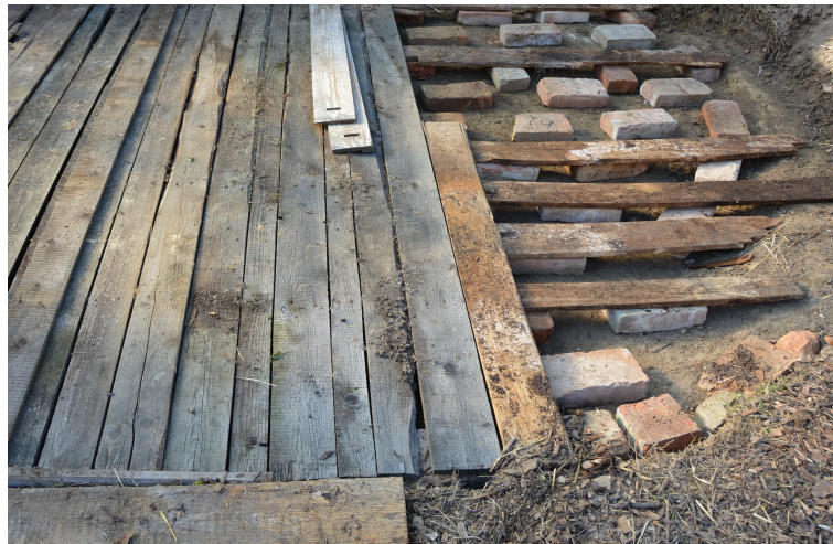
Figure 9. Compost floor—underlying bricks and wooden panels provide thermal insulation of the composting material from the ground. Figure shows the construction in progress that is almost ready for installation of waterproof plastic layer.
