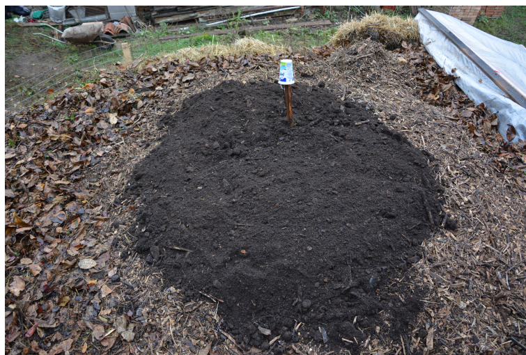
Figure 12. A compost biofilter cover layer of about 20–30 cm is applied on top of the permeable layer covering the heat exchanger.
