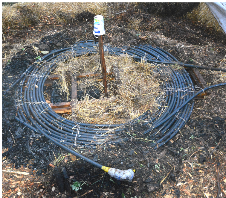
Figure 5. The heat exchanger is gradually covered with porous materials. Note that the cavity is formed underneath the piping, allowing condensation to happen. The temperature sensor for a compost core is installed inside the yellow tube while still uncovered. The wire is hidden under the white cup.
