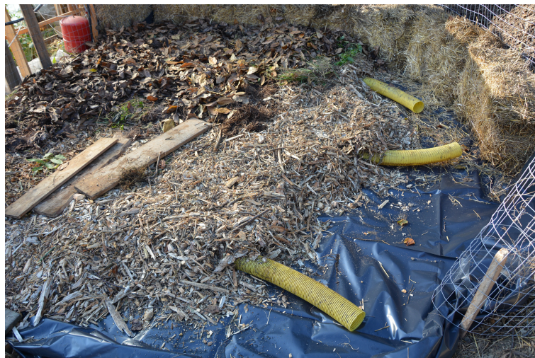
Figure 10. Waterproof plastic layer and perforated tubes covered with the aeration plenum layer (woodchips).
