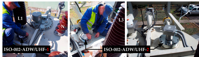
Figure 30. The installation of the active dielectric windows with UHF antennas (ISO-002-ADW/UHF-1 and ISO-002-ADW/UHF-2) in the revision holes of the upper cover of the 31.5 MVA power transformer tank.
