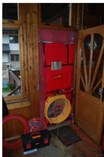
Figure 7. Envelope airtightness test performed on the Stara Polana building. Location of the Blower Door device in the entrance door. Reproduced from [22].
