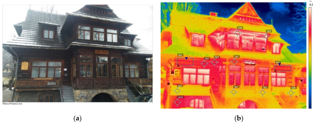
Figure 6. (a) Front facade. (b) General thermovision analysis of the Stara Polana building using a FLIR camera.
