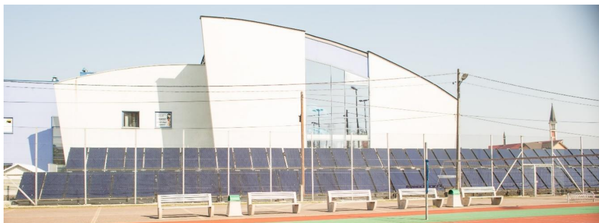
Figure 1. The flat plate collector (FPC) installation in Brzesko.
