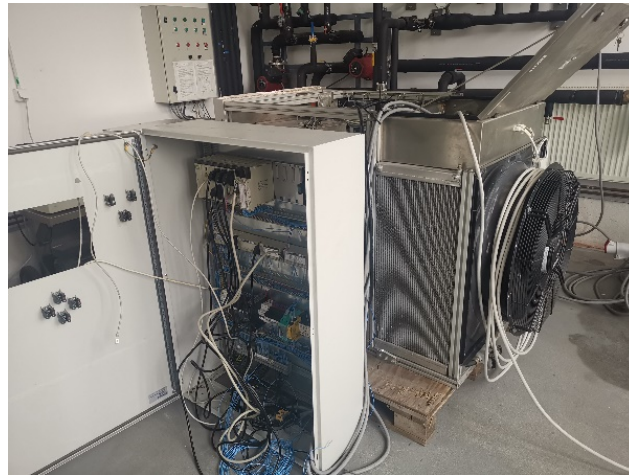
Figure 11. CPU and automation panel.
