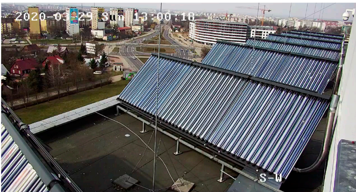
Figure 2. Evacuated tube solar collectors connected in series of three panels grouped into five subarrays.
