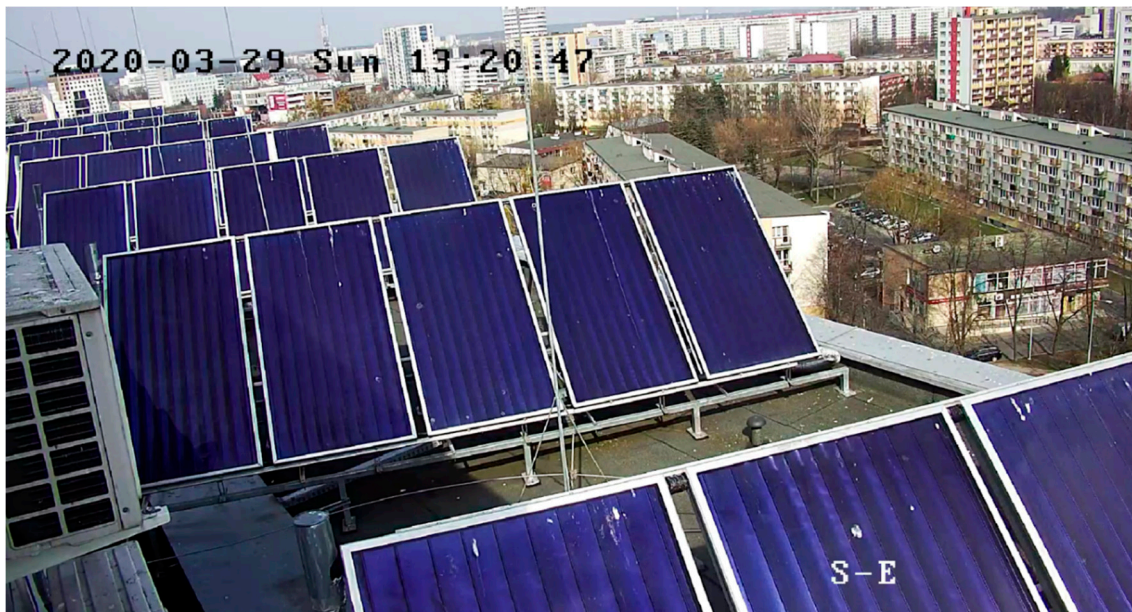
Figure 1. Flat plate solar collectors connected in series of five panels grouped into seven subarrays.
