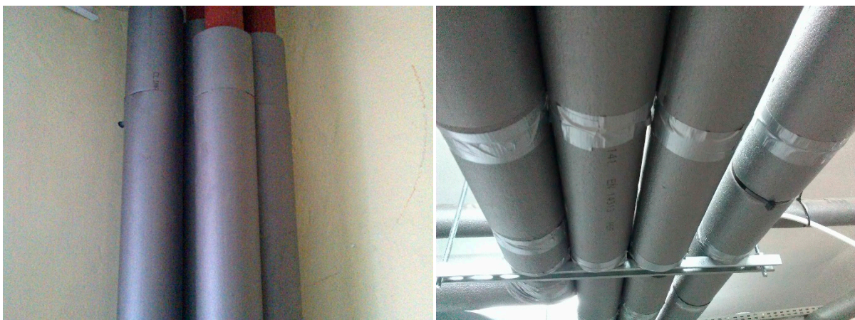
Figure 4. Thermal insulation on pipes under consideration (photo taken by the author).
