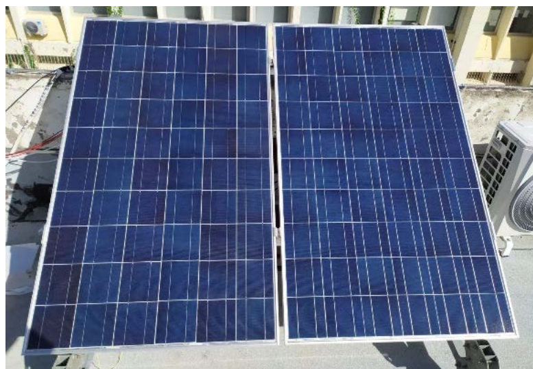
Figure 10. Photovoltaic panels PV_1 and PV_2 used for the experiments.
