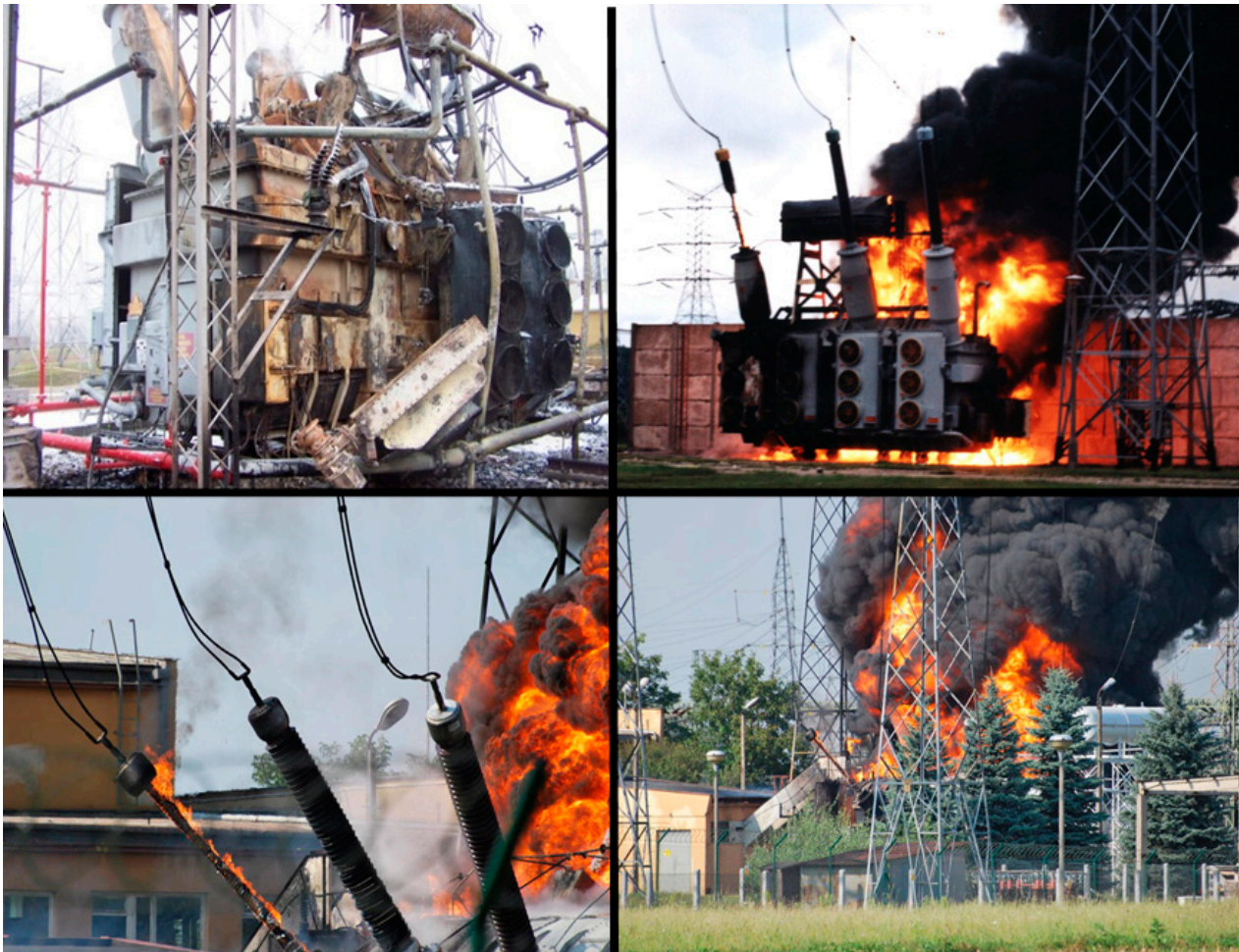
Figure 2. Examples of catastrophic failures of high power transformers initiated by the failure of a bushing.
