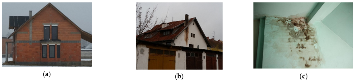
Figure 5. Consequences of inadequate protection of external and internal chimney walls (a,b) elevation, (c) inside.
