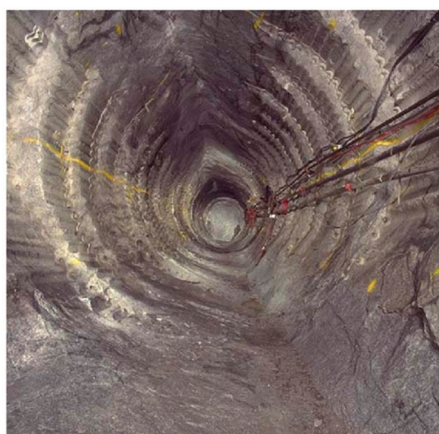
Figure 4. Damage profile of a tunnel excavated at depth 420 m within massive hard rock in Canada [35].
