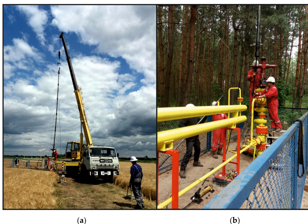
Figure 1. Sampling of bottomhole samples; (a) assembling lubricator at B-24 well; (b) pulling out the bottomhole samplers from the B-22 well lubricator.
