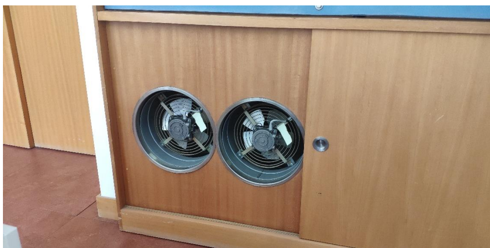
Figure 10. Office earth tube opening.
