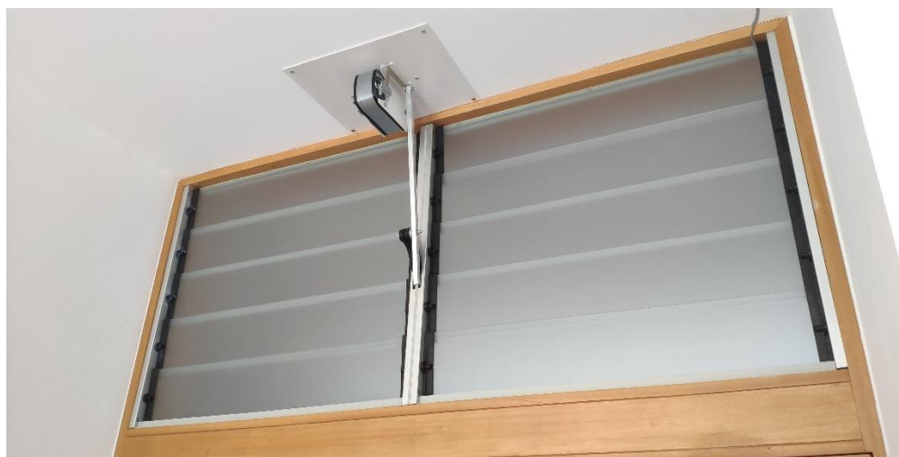
Figure 9. Over-door air vent.
