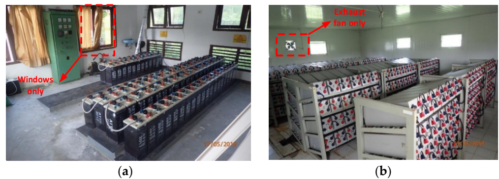
Figure 8. Battery rooms; (a) PV site 1; (b) PV site 14.
