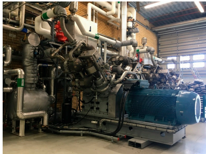
Figure 2. The highlift Stirling-cycle-based heat pump (SC HP) developed by Olvondo Technology, Norway and being used by the pharmaceutical company AstraZeneca, Gothenburg, Sweden.
