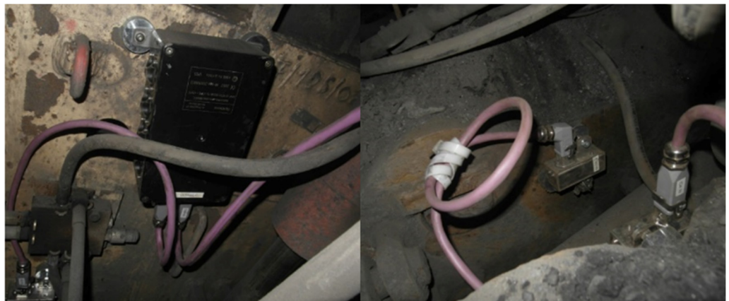
Figure 6. SSMS system components: Central unit SSMS-C and Inclinometer SSMS-I mounted on the shield support.
