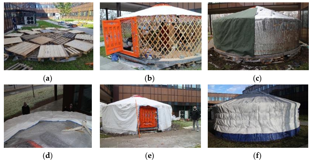
Figure 3. The materials used in the yurt tested in Cracow, Poland (photographs taken by Piotr Śliwinski during construction of Mongolian yurt in Cracow in 2020). (a) wooden pallets supporting yurt; (b) walls of the yurt and the first internal layer, white fabric; (c) the second layer, aluminum films with PE foam and spacer strips of polystyrene, the third layer green tarpaulin; (d) fourth layer, bubble foil; (e) the fifth layer, white protective synthetic material; (f) final view of modified yurt.
