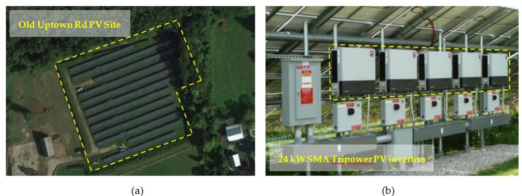
Figure 10. Field Demonstration. (a) Aerial View of the Old Upton Rd PV Site. (b) PV Inverters at the PV Site.
