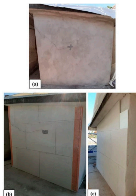
Figure 2. Selected test rooms in their original state (a) and during aerogel panel installation (b,c).
