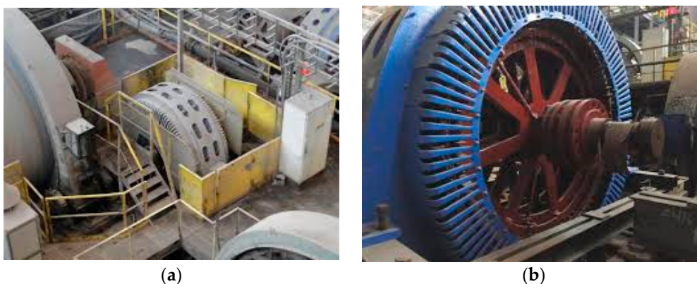
Figure 2. Ball mill drive system with low-speed SAS motor without intermediate gearbox: (a) prior to modernization, (b) after modernization on the right [34].
