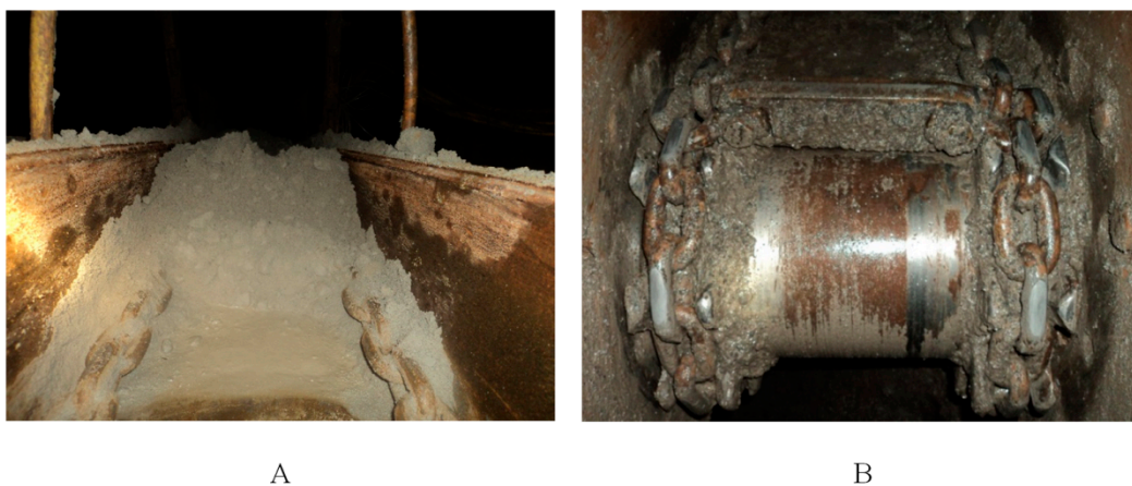
Figure 1. Examples of the presence of dry mineral abrasive (A) and mixture of water with abrasive (B) on transmission elements in corridor conveyors.
