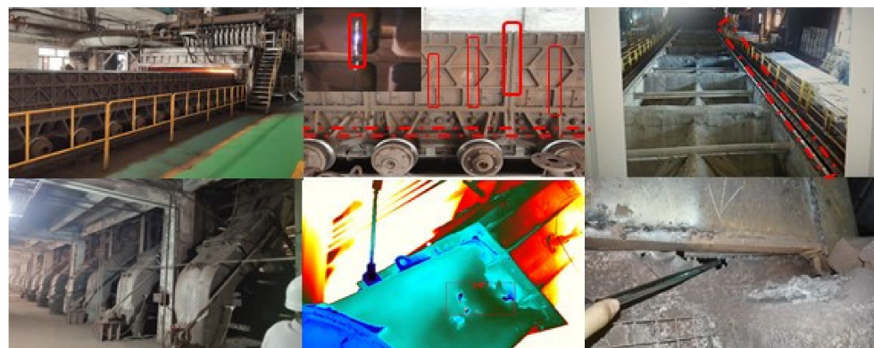
Figure 2. Some typical leakage in region A.
