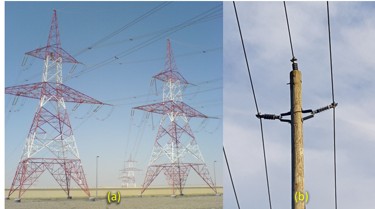
Figure 10. Photos of (a) a 220-kV overhead transmission line where outdoor insulators are employed to electrically isolate the conductors from the grounded towers, and (b) is a 12.47-kV wooden post using polymer insulators for isolating the conductors from the pole.
