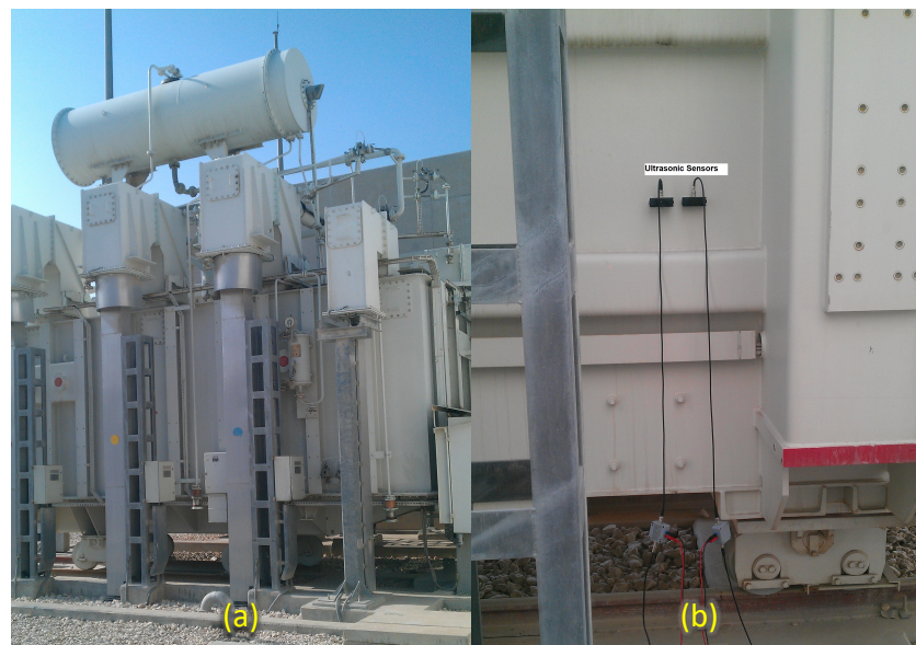
Figure 9. (a) A photo of a power transformer, (b) acoustic sensors installed on the tank of a transformer.
