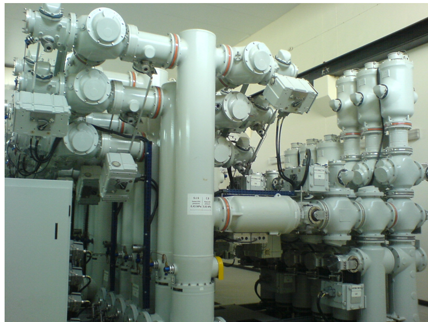
Figure 8. Gas insulated switchgear.
