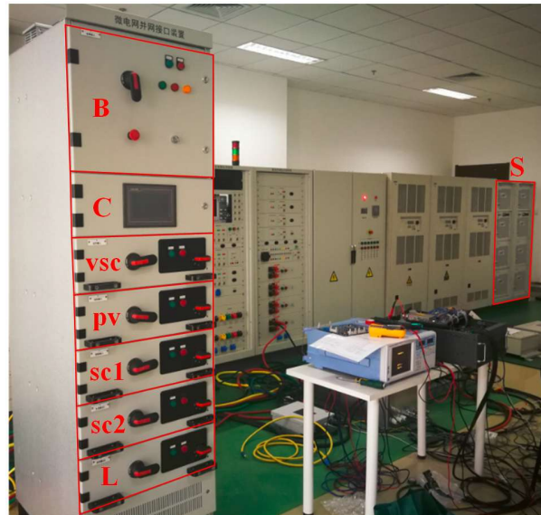
Figure 14. DC microgrid experimental platform.
