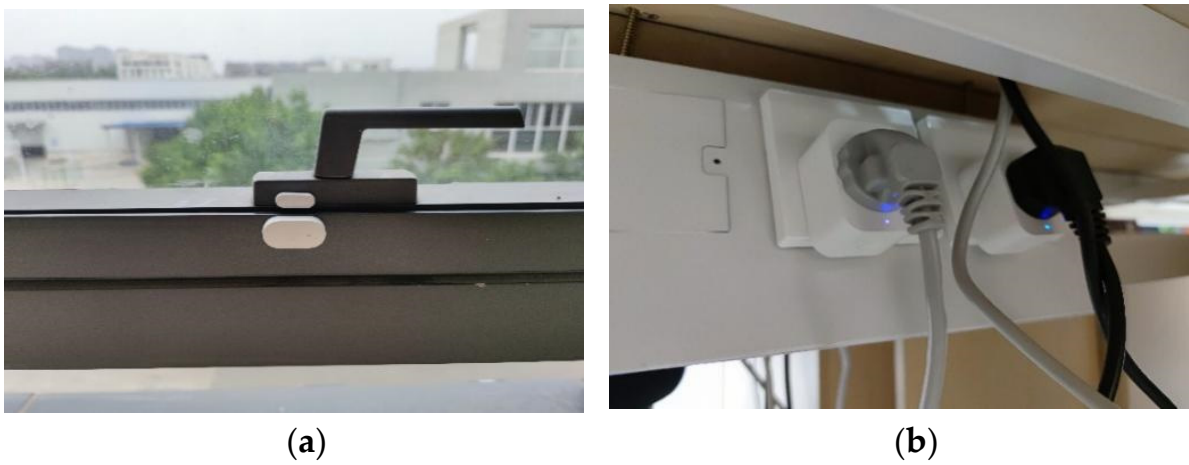
Figure 7. (a) Door and window sensors, (b) smart sockets.
