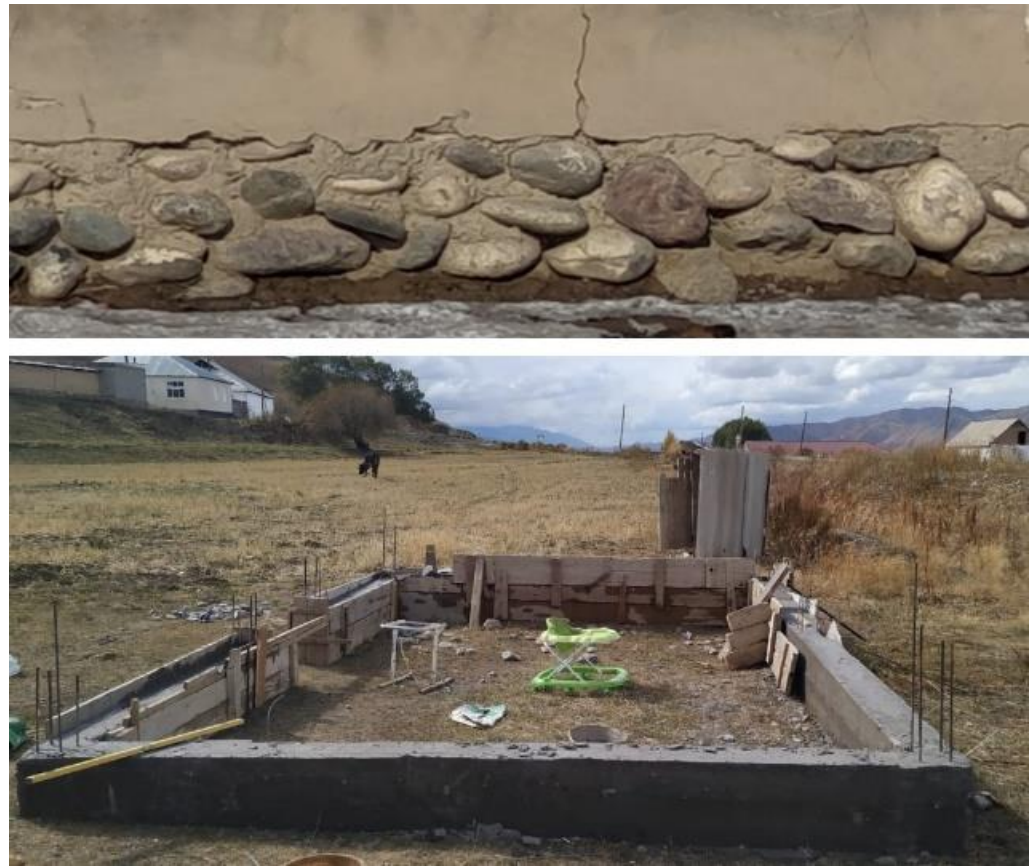
Figure 8. Foundation with the stone ( top ) and foundation with the concrete frame ( bottom ).
