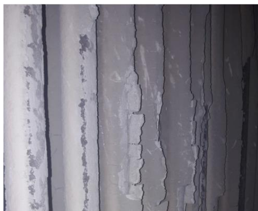
Figure 18. Slag deposits on the water wall surface.
