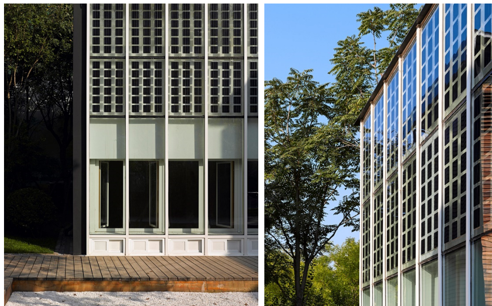
Figure 3. A photovoltaic double skin-façade in Beijing [10].
