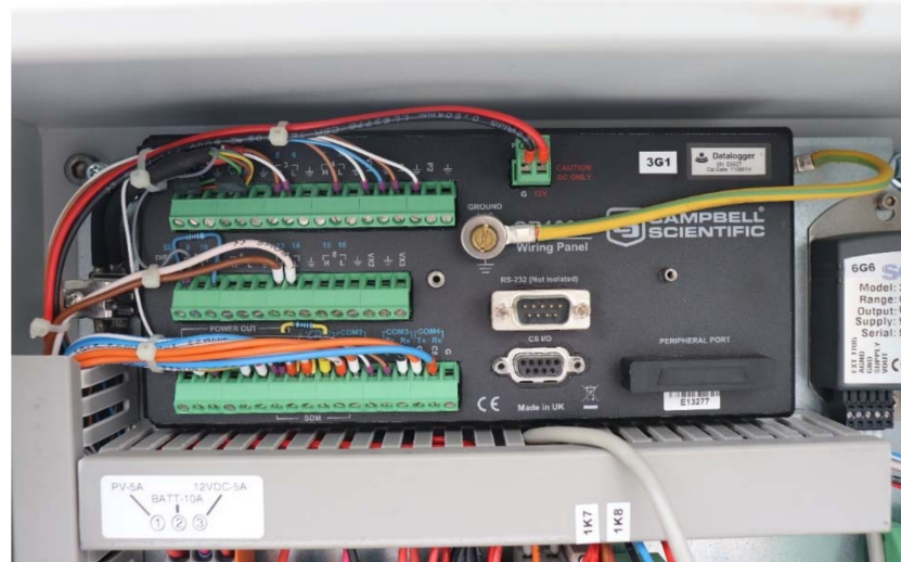
Figure 4. CR1000 data logger installed at UET Peshawar’s weather station.
