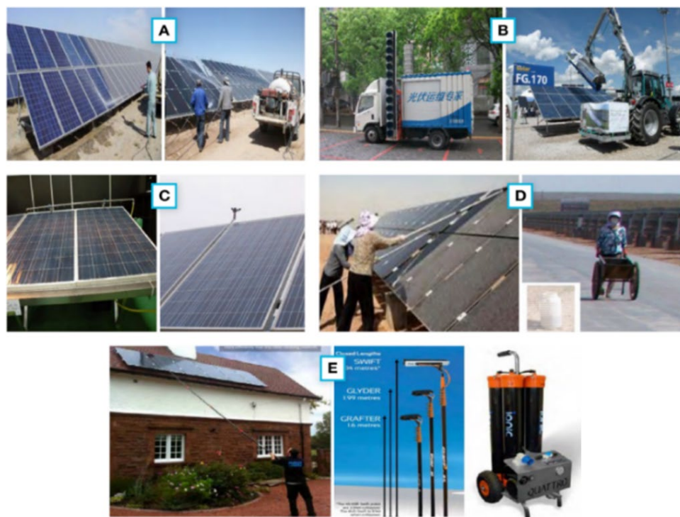
Figure 9. Popular PV panel cleaning methods in the desert. (A) Spraying water; (B) special cleaning vehicle; (C) water pipes; (D) human method; (E) special pressured water brush.
