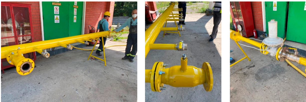
Figure 5. Experimental stand structure for losses due to ill-fitting (1—pipe coupon with a minimum diameter of 150 mm and a length of 6 m, 2—pressure transducer, 3—data acquisition system, 4—pressure-time recording system, usually with PC, 5—flow meter with rotating pistons, 6—gas source, 7—temperature transducer, 8—faucet, 9—pressure gauge, 10—various types of equipment) (source: authors based on the real analysed equipment).
