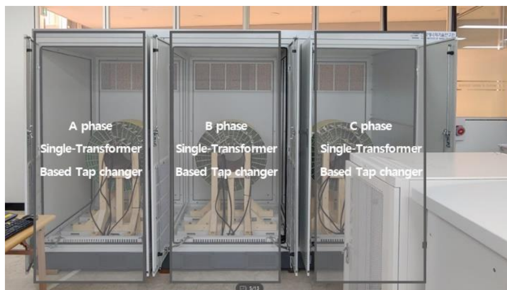
Figure 16. A 30 kW-scale LVRT/HVRT facility.
