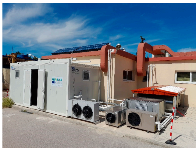
Figure 1. The installed energy system with outdoor components and its containerized control room.
