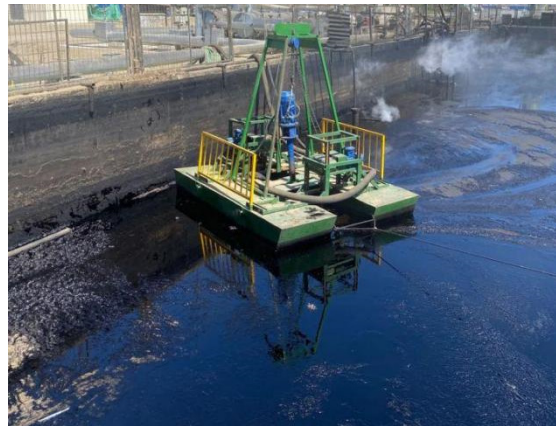
Figure 1. Picture of oily sludge settling tank in an oilfield.
