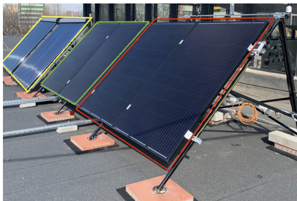
Figure 4. Photograph of the panels installed on the roof, showing ST panels in yellow, PVT panels in green, and PV panels in red [20].
