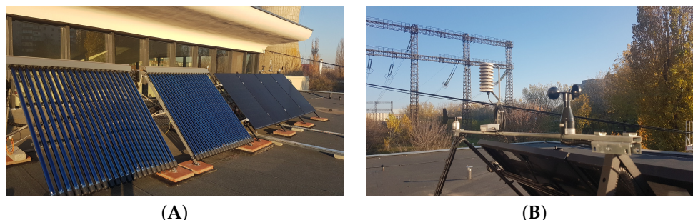
Figure 2. Photographs of (A) the installed panels and (B) the meteorological station [20].
