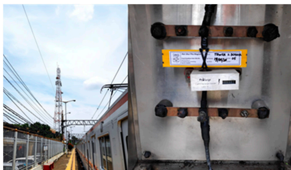
Figure 12. Installation of measurement system in a telecommunication tower.
