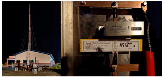
Figure 19. Installation of measurement system in a mobile lightning protection system for a mining area.
