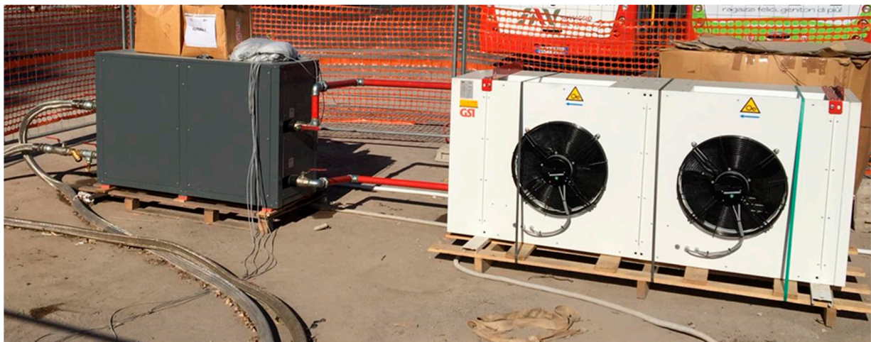
Figure 3. Dry cooler (right) and management and control apparatus (left).
