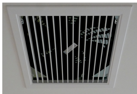
Figure 10. Detail of an individual ceiling fan in the LRAD building. An adjustable grid was applied below the fan to allow focusing the air movement to the workplaces.
