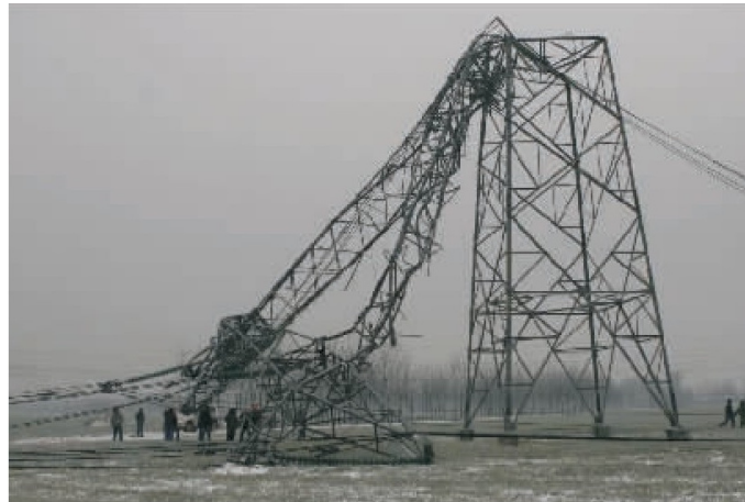
Figure 1. The collapse of the power grid tower was caused by the snow and icing disaster [10].
