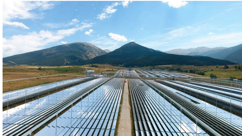
Figure 1. Photo of the eLLO solar power plant.
