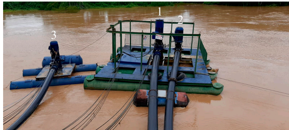
Figure 2. Elevated Pumping Station II, Rio Branco, Acre, consisting of a set of vertical turbine-type pumps. Note: 1—Pump 1; 2—Pump 2; and 3—Pump 3.
