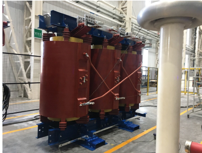
Figure 24. Actual arrangement of transformer voltage test.
