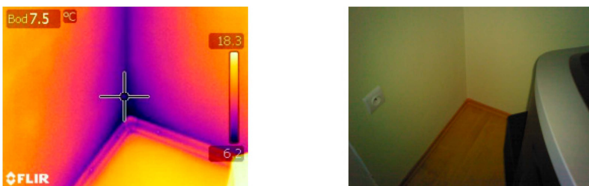
Figure 8. Thermal camera image showing deficiencies within the building envelope [authors].
