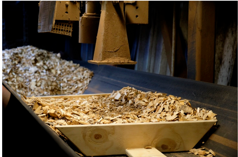
Figure 10. The MW-based system for in-line measurements of the water content of woodchips. The system is installed at the conveyor belt feeding the boilers. In the photo, the belt is stopped for the calibration measurements.
